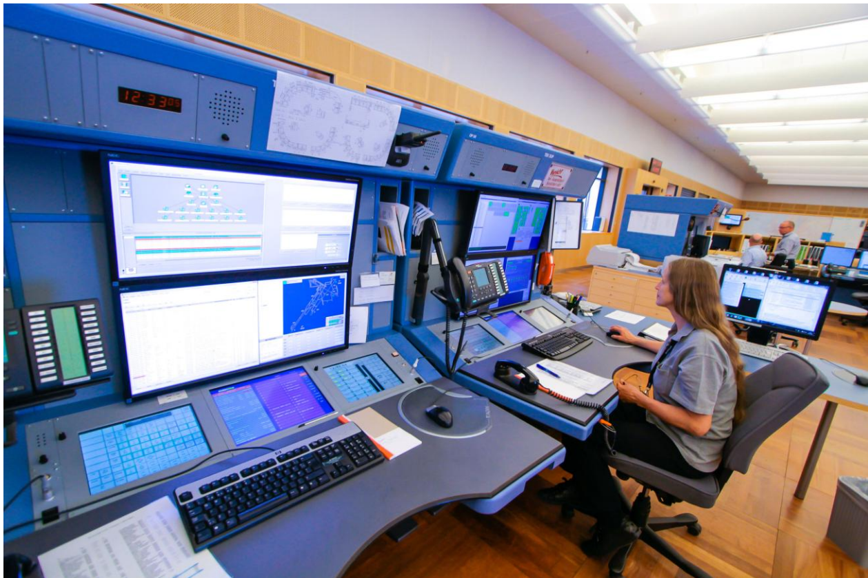
Figure 10: ATSEP SMC. Picture courtesy of Entry Point North.
